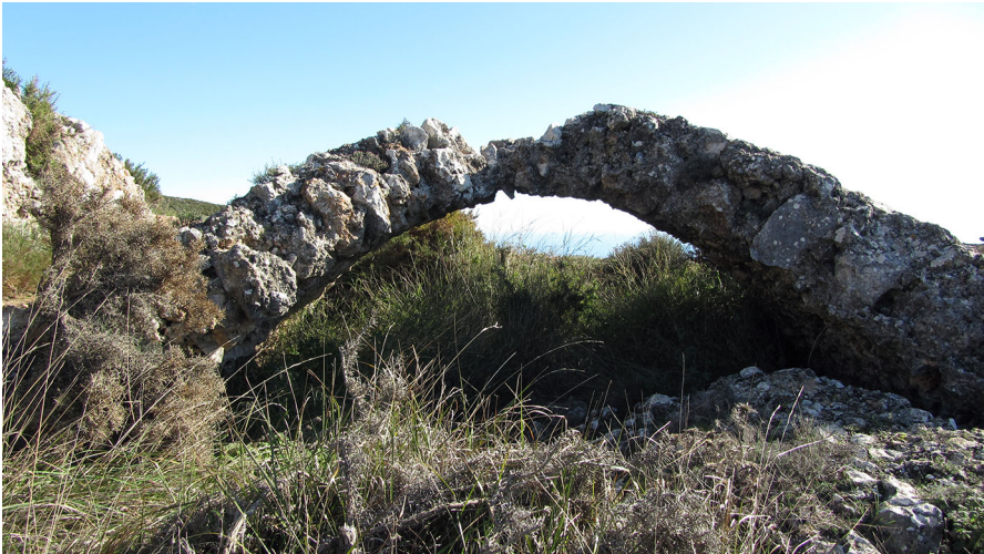
Fig. 11 One of the collapsed vaults of the access level. The ruins show clearly the building technique used for structural elements, which of course could not be built with rammed earth. Photo by Silvia Bertacchi
