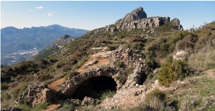
Fig. 8 The collapsed vault covering the dugout of the western bastion seen from the ancient access to the fort. Photo by Silvia Bertacchi
